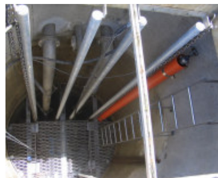
Pump Station Level Measurement with Ultrasonic (in orange pipe)
