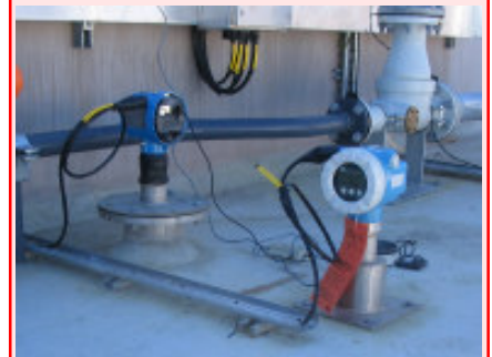
Commissioning of Micropilot Radar and Prosonic Ultrasonic Systems on WWTP Lime Batching Tank
