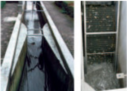
Typical Prosonic S applications: Open Channel Flow Measurement and Screen Monitoring / Control
