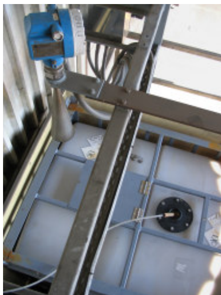
FMR240 Micropilot M mounted above IBC
