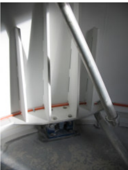
Inside the silo base showing one of the Loadcell Mounts and Strengthening Plates
