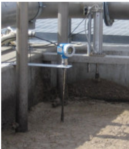
Levelflex FMP40 installed at NSCC - WWTP
