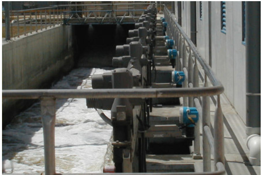
Endress+Hauser Prosonic M FMU40 Ultrasonic Level Transmitters at Manukau WWTP "Photos courtesy of Watercare Services Ltd"
