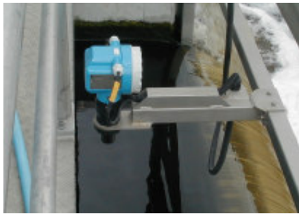
FMU40 mounted on the penstock weir
