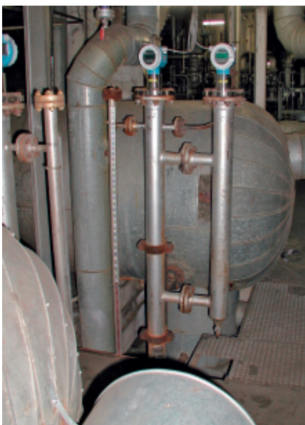
Levelflex M on low pressure heater
