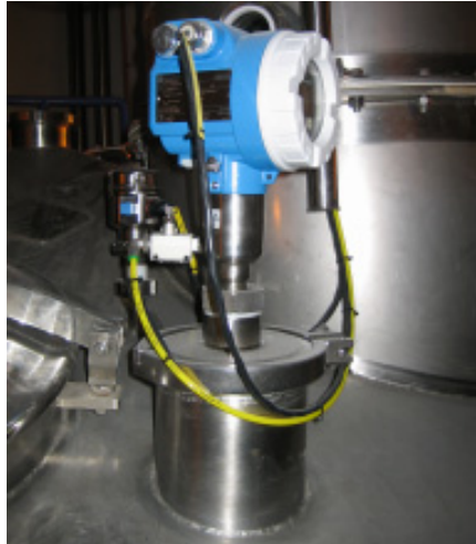
FMR250 Radar on Milk Powder Silo
