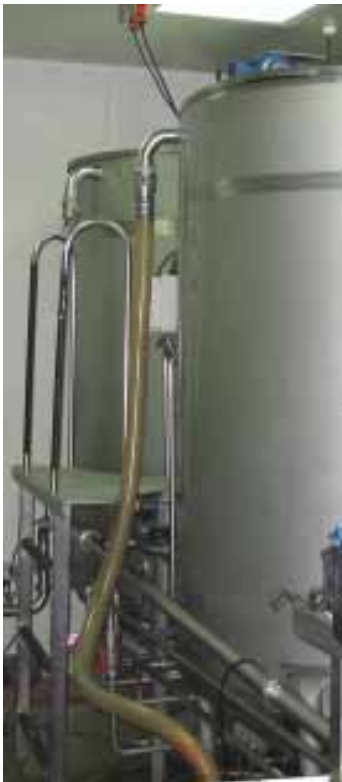
Liquid Storage Tanks
