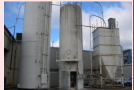
DSM Mounts on 30t skirted Flour Silo
