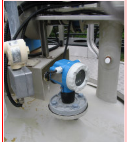
Prosonic Ultrasonic System on WTP Sodium Hypochlorite Tanks
