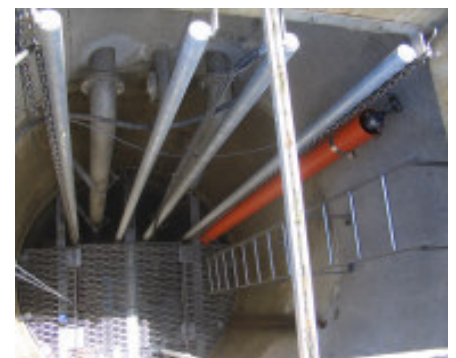
Pump Station Level Measurement with Ultrasonic (in orange pipe)
