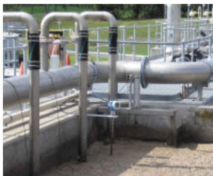
Levelflex Guided Radar in Activated Sludge Reactor
