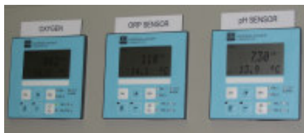
Recent Liquisys M Installation for Dissolved Oxygen, ORP and Memosens pH
