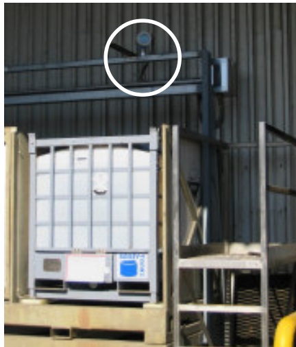
IBC at Amcor - FMR240 circled
