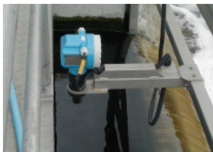
FMU40 mounted on the penstock weir
