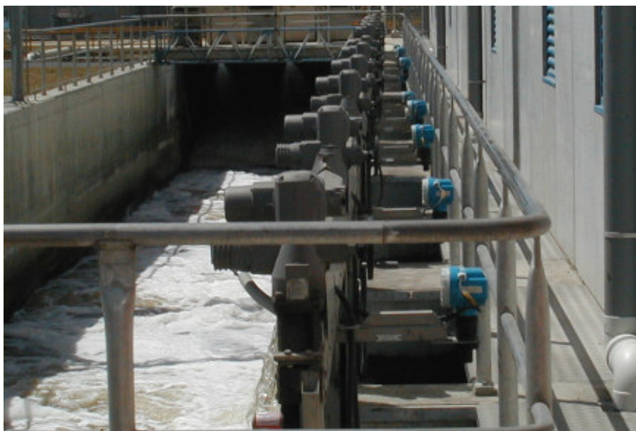
Endress+Hauser Prosonic M FMU40 Ultrasonic Level Transmitters at Manukau WWTP "Photos courtesy of Watercare Services Ltd"
